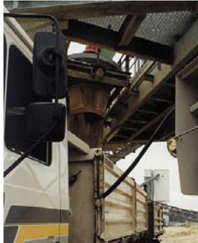
Continuous Flow Mixer integrated in truck loadout station
