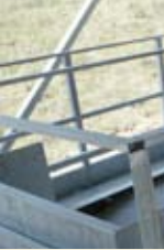
Reclaim Weigh Belt Feeder
